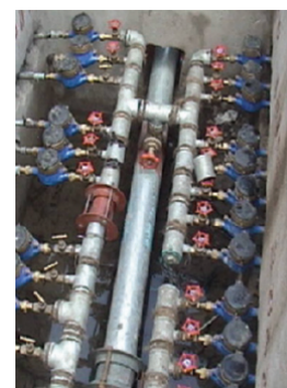
Figure 2.13: Water meter chamber, Mukuru, Nairobi
